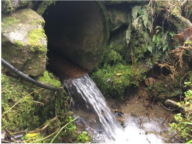
Perched culvert pipe
